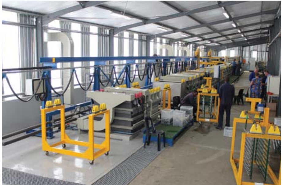
The new chrome plating plant is capable of processing 200 000 components per month with an OEE of 80%. PDC is not a jobbing operation and has reserved the full capacity for Cobra's production
